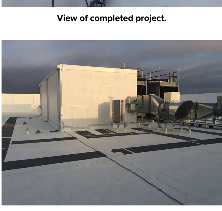
New high density cover board installation set in low rise foam adhesive 4" on center.
