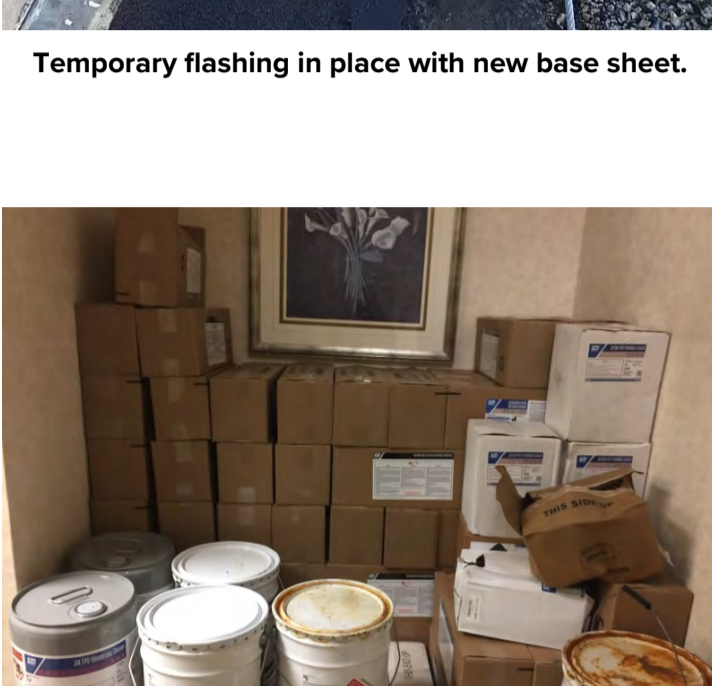
The existing roof deck has been indicated to be unsafe for foot traffic in this area.
