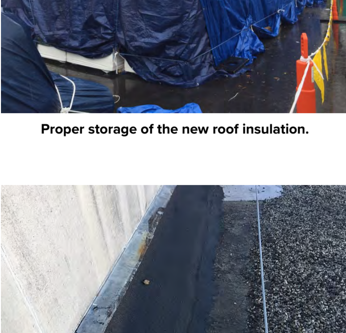
Prepped around the walls to have ready for asbestos guys to remove wall flashing.
